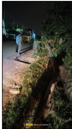
Street pole damage- Near Manjushree Road
