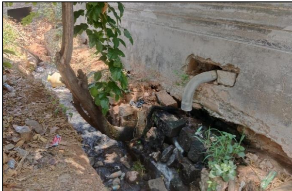
Discharging Waste water - near Rajhans backgate road
