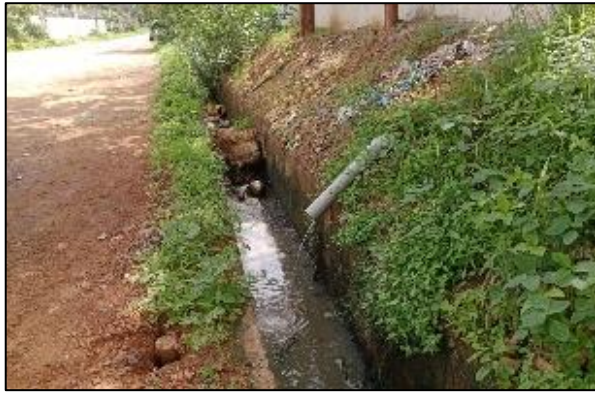
Discharging Waste water – Ambience Road
