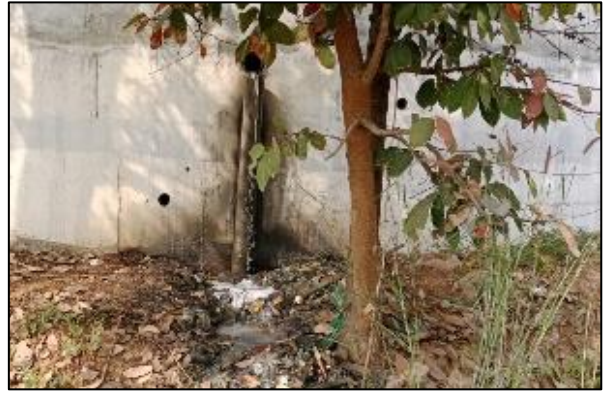
Discharging Waste water - Beside Saree Udog Industry
