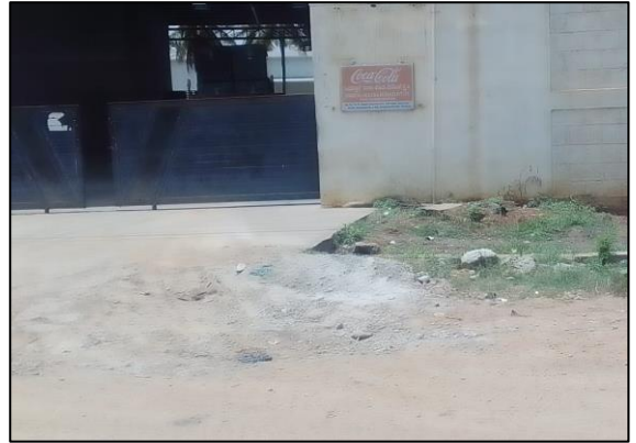
Dumping construction material – near Manjushree Road
