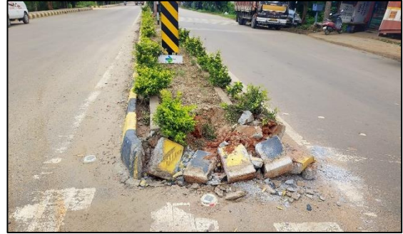
Kerbstone damaged – near Shyanamangala Circle
