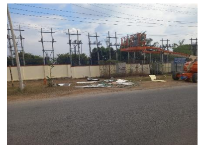
Waste dumped near M/s KPTCL Substation
